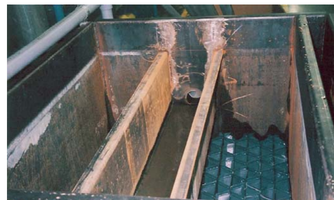
Top View of CLARIFLO Tank with Tube Media Installed
